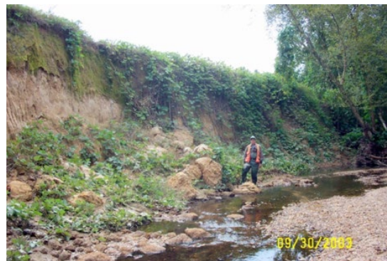
Figure 24. Examples of Mass Wasting or Bank Failure
