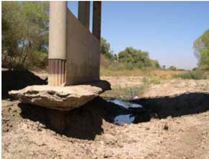
Figure B3.8. Main Street bridge showing exposure of bridge pier foundation due to bed lowering.
