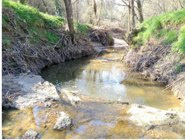
Figure B4.7. Arcade Creek site 13. Exposed tree roots in banks, leaning tree trunks, small width to depth ratio, and vertical drop at concrete apron in foreground are collectively diagnostic for channel incision.
