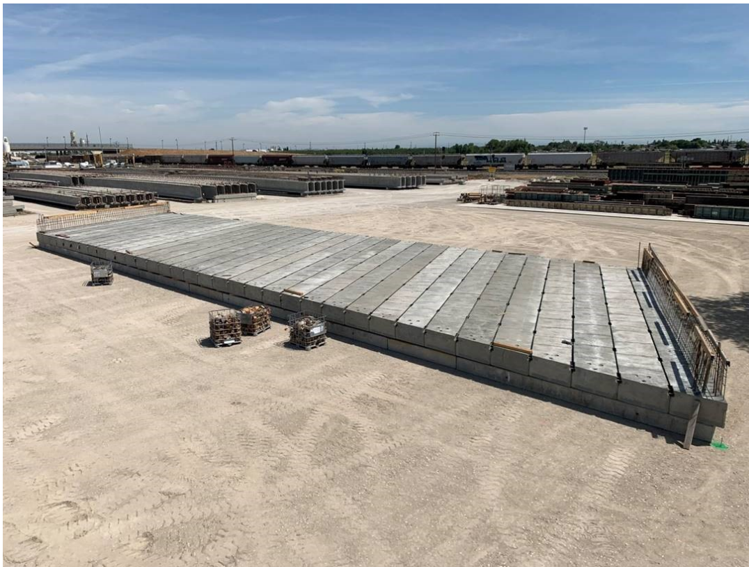
Figure 4.9.8-1 Preassembled Precast Concrete Box Girders Prior to Shipping, 21 st Ave UC (Replace), Contract No. 03-0H3424.
