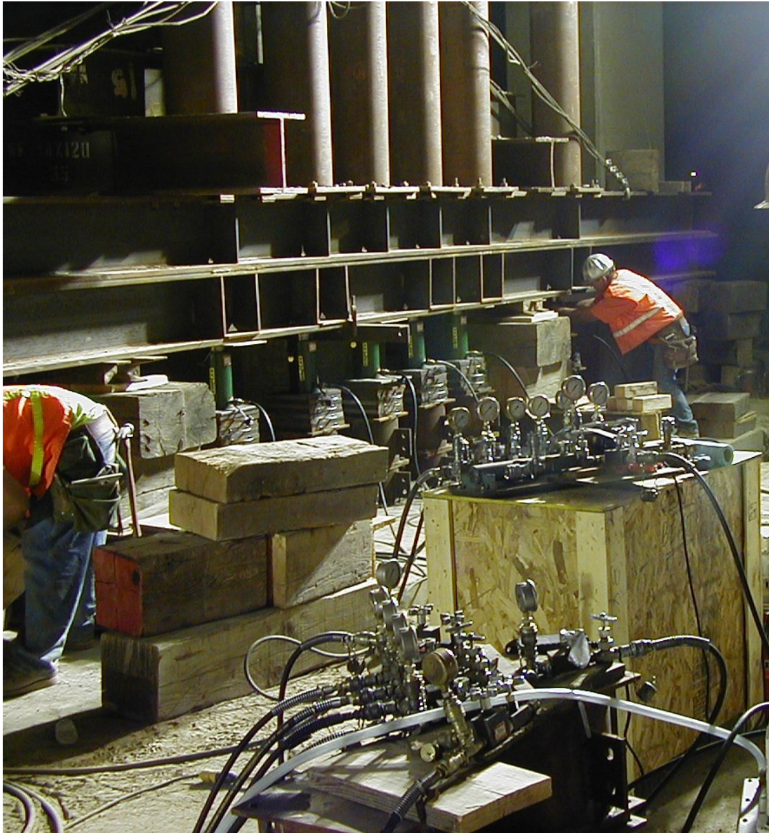
Figure 2. A jacking manifold used to split the hydraulic line to individual jacks. Note that each jack has a dedicated control valve and pressure gauge.
