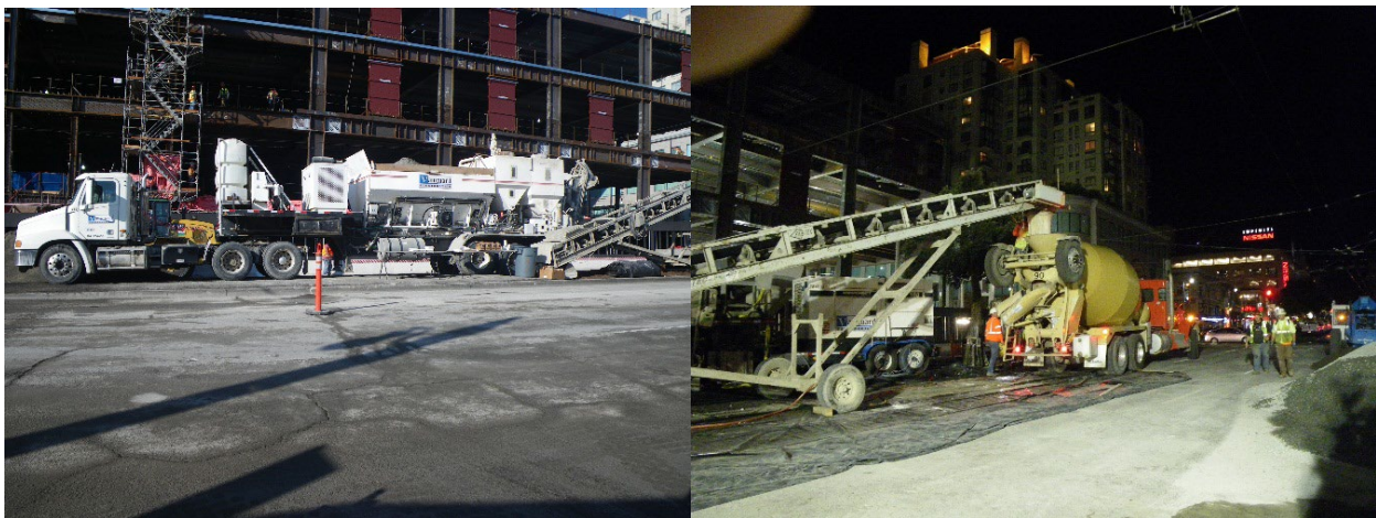
Figure 2. Volumetric Mixer belted into Drum Truck
