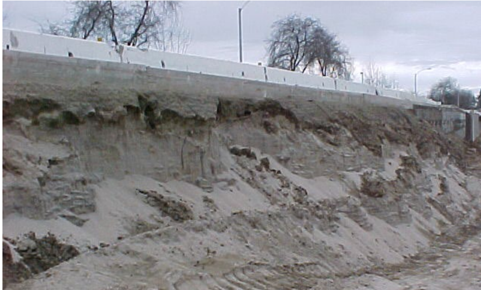
Figure 1. Native sandy silt material that will not maintain a vertical stable cut.
