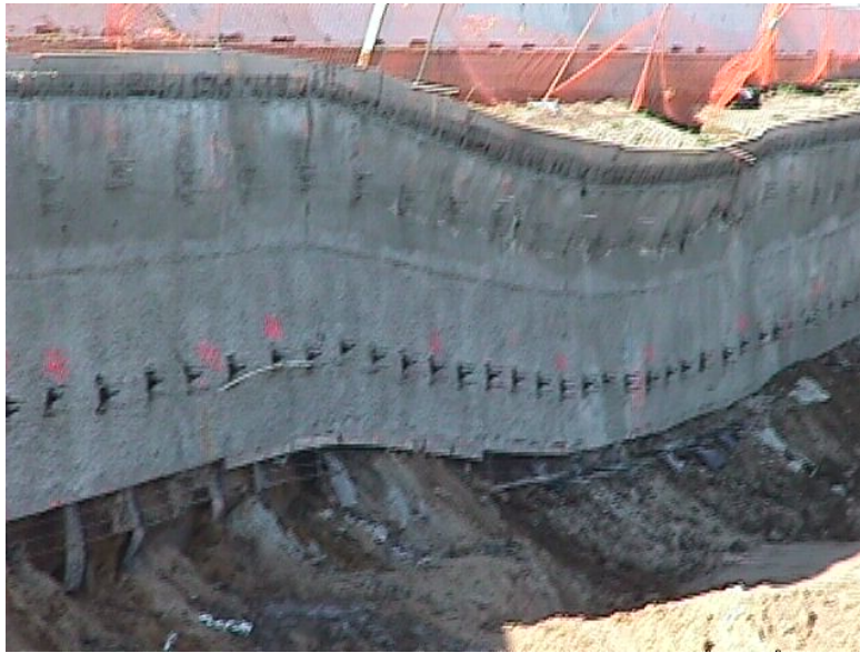
Figure 7. Wall collapsed due to progressive loss of material from behind the wall, noted in the previous pictures. Notice the deteriorated berm and loss of material
