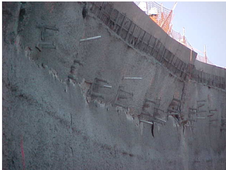
Figure 8. With the loss of the supporting soil behind the wall, the wall failed similar to a beam in bending. The top portion of the wall buckled outward and broke.
