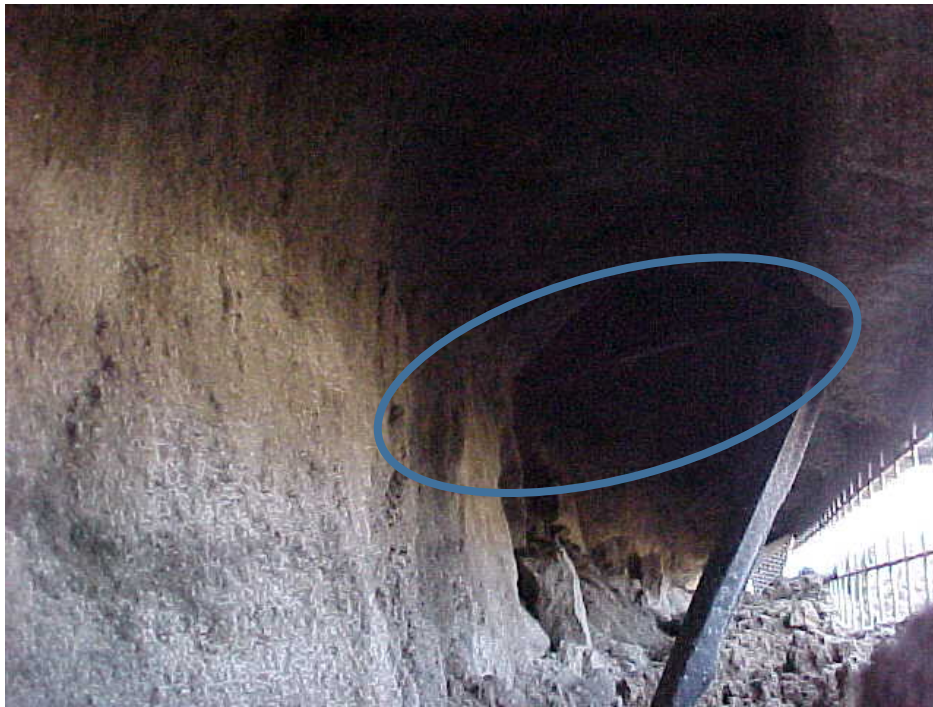
Figure 6. Picture from inside and behind shotcrete to illustrate the amount of material loss. Note the exposed soil nail from the previously completed row above.
