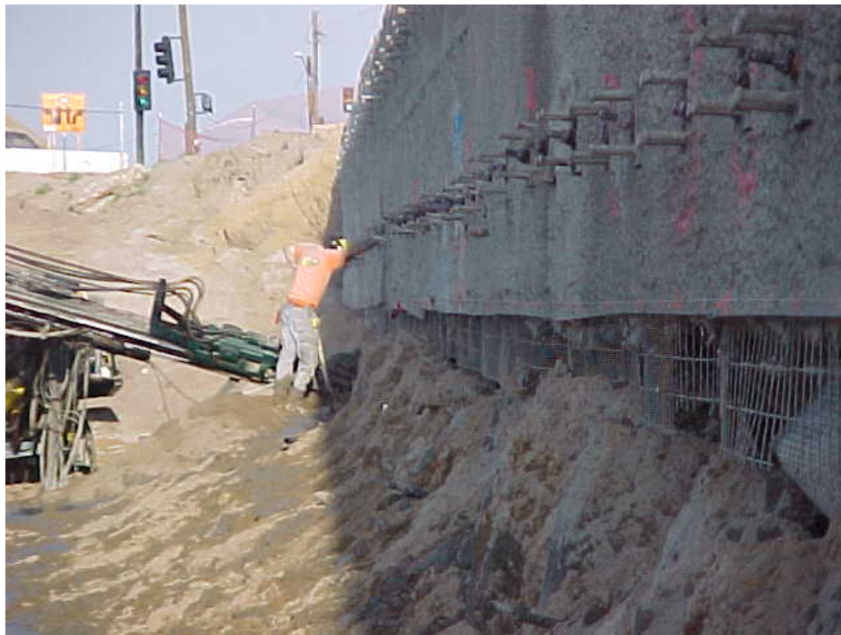
Figure 4. Improper berm and native sandy material sloughing on Friday from behind the previously constructed 2 layer/rows of soil nails.
