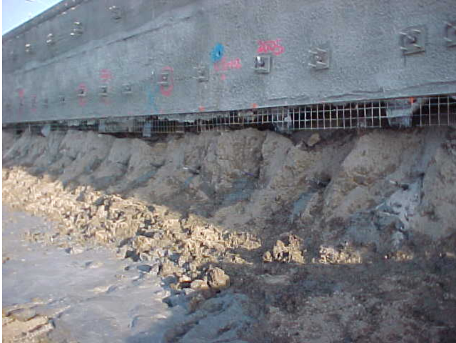
Figure 5. As work progressed through the day and afternoon more material sloughs from behind the wall due to construction activity and loss of moisture.
