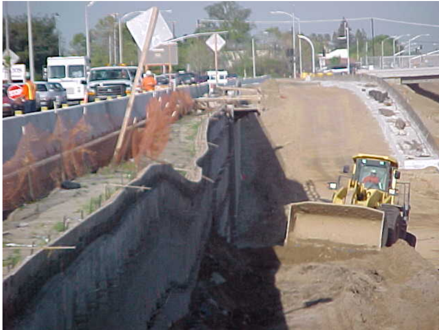
Figure 9. Illustrating the magnitude of material loss due to wall face instability and potential safety hazard for the travelling public. The berm being placed is to stabilize the failed section to prevent further collapse.
