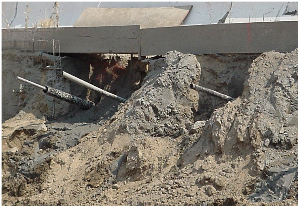
Figure 2. Another example of wall face instability due to sandy material.
