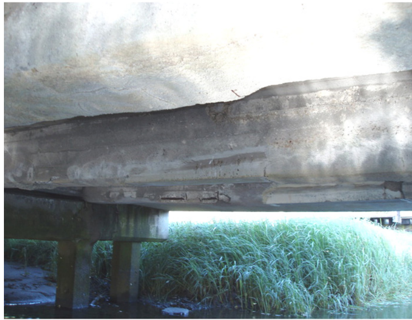
Figure 1-5. Corrosive Girder Spalling.
