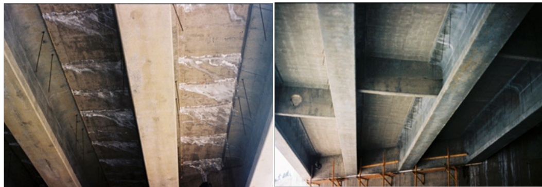
Figure 1-4. Deck Cracks Before and After Use of SRA.
