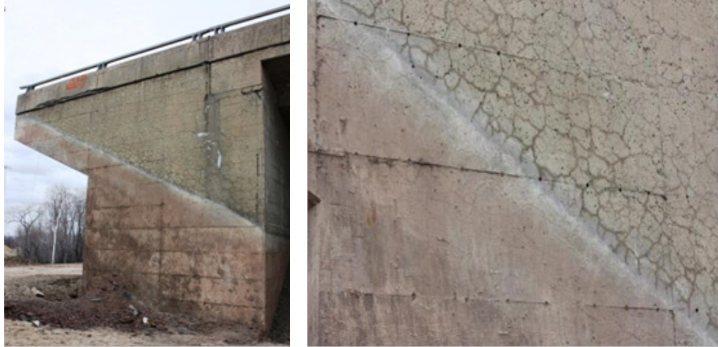
Figure 1-7. Concrete Deterioration Due to Alkali-Silica Reaction 4 .
