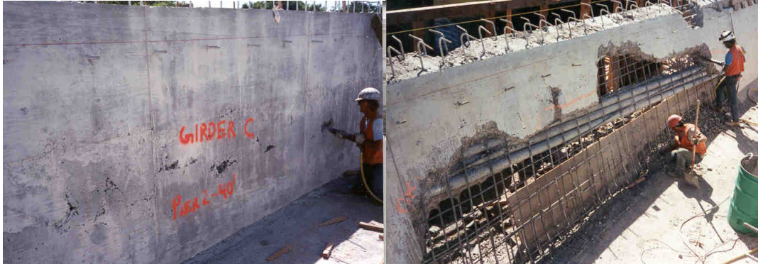
Figure 6-2. Rock Pocket Damage.
