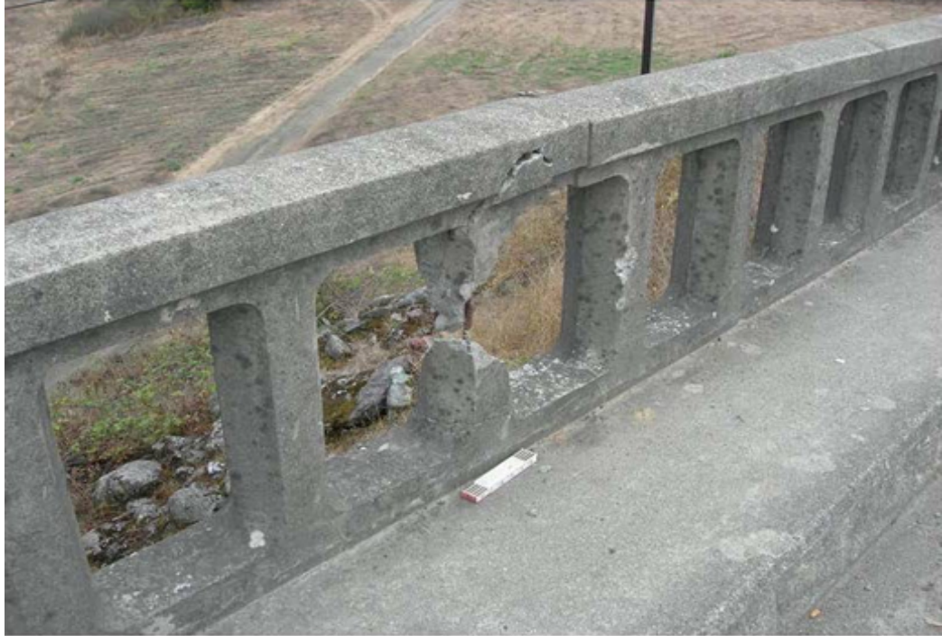
Figure 6-6. Surface Spalling Caused by Vehicle Impact.
