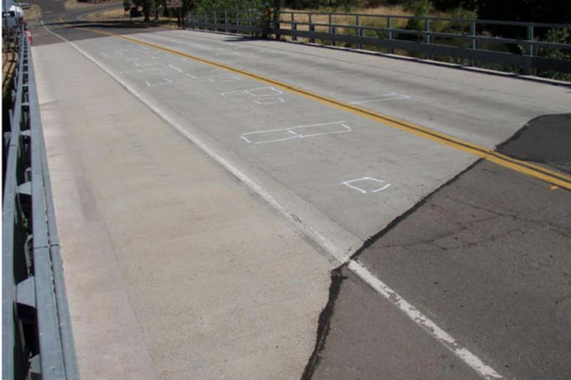
Figure 6-7. Delaminated Deck Surfaces Identified for Replacement.
