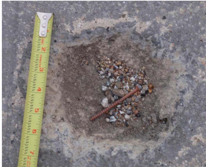
Figure 6-4. Severe Bridge Deck Scaling, Small Pothole.
