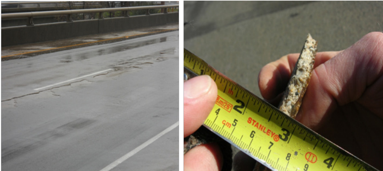
Figure 6-19. Polyester Overlay Spalling.
