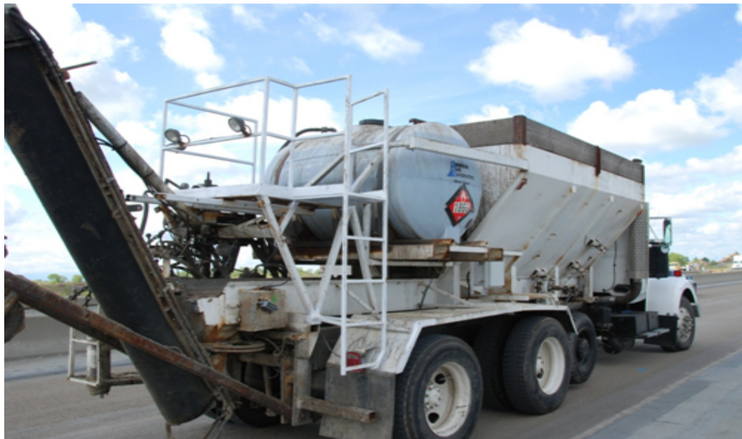
Figure 6-16. Volumetric Operation (Note HAZMAT Placard ID # 1866).
