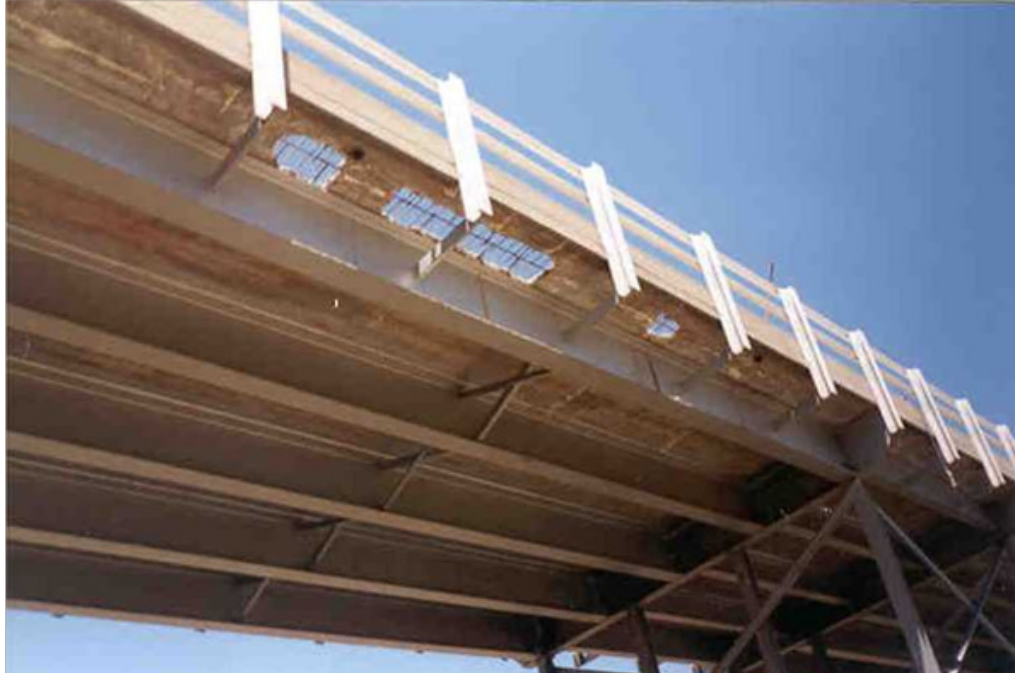
Figure 6-1. Initial Damage Assessment.
