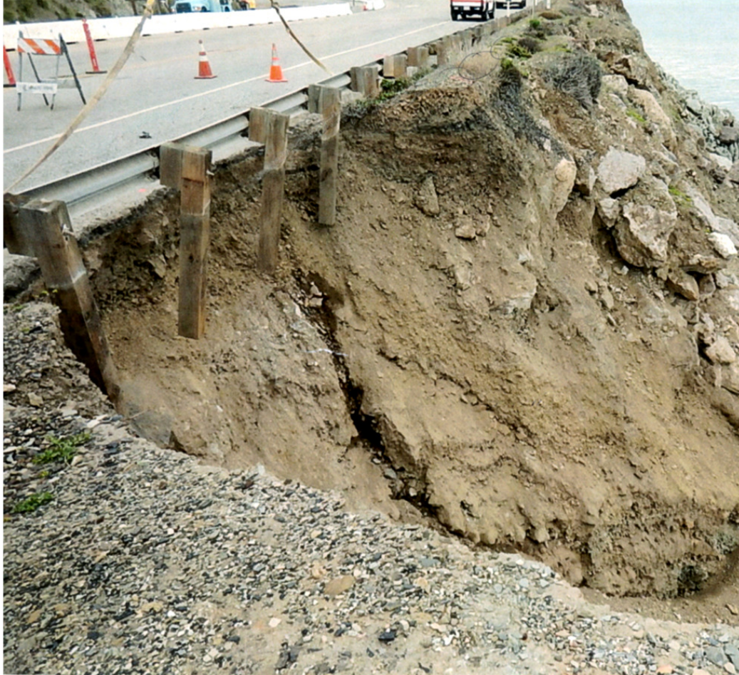
Storm damage to the Pacific Coast Highway shoulder at Sycamore Cove day use beach at Point Mugu State Park in the Santa Monica Mountains
