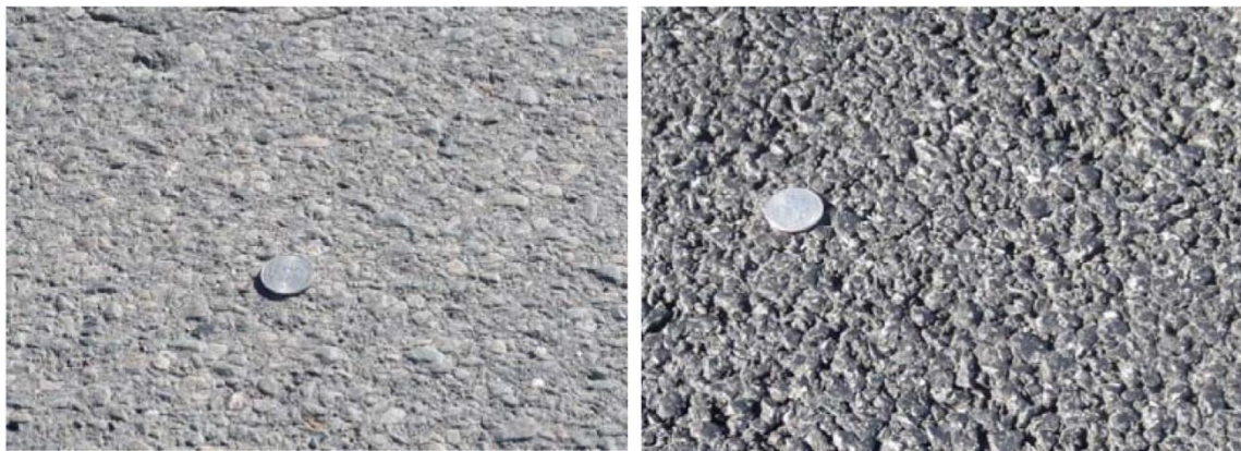
Figure 6-11: Photographs of San Pedro Road Pavement Surfaces
