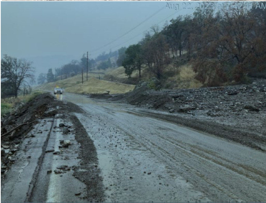
02-SIS-96 – Typical Damaged
