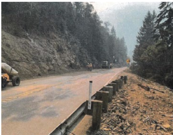
01-DN-199 – Typical wildfire damage
