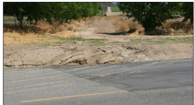
Figure 3.31: Access road drainage problems (note patch).
