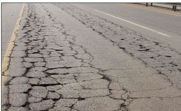
Figure 3.34: Loose blocks in severe alligator cracking.
