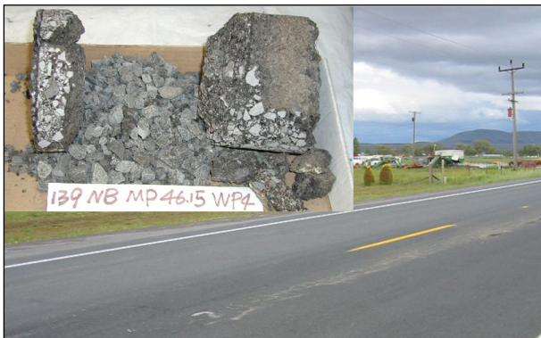
Figure 2.5: Example of fines pumped through alligator cracks from stripped asphalt layers. (Core photo in insert)
