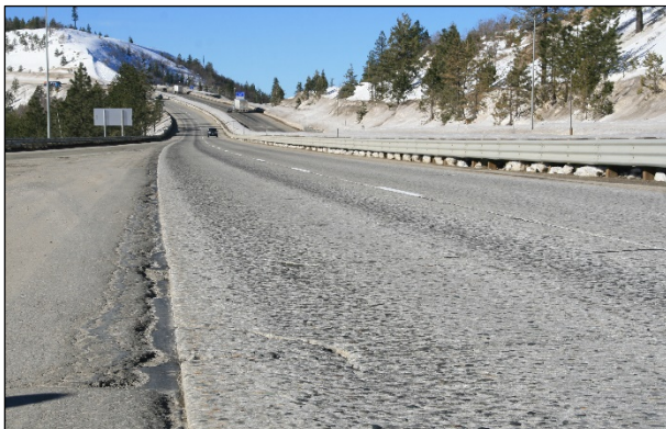
Figure 3.20: Wheelpath rutting from chain wear on jointed plain concrete pavement.
