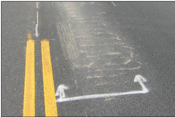
Figure 2.3: Example of pumping.
