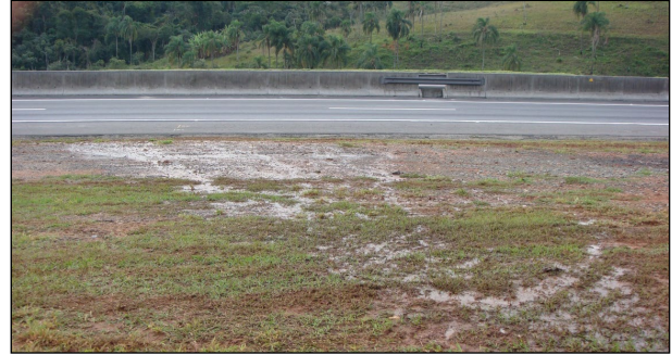
Figure 3.33: Water flowing downslope into the road.
