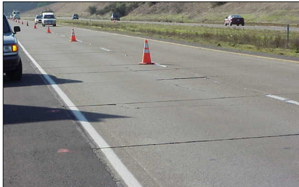
Figure 2.7: Example of faulting and transverse and corner cracks on concrete pavement.
