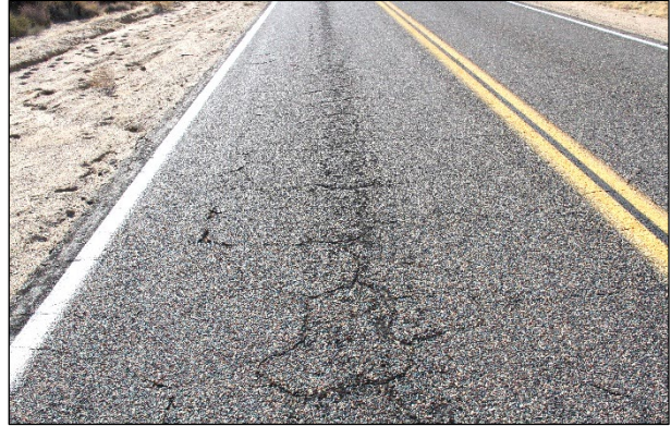
Figure 3.6: Oxidative-aging cracking in random pattern.
