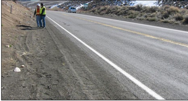
Figure 3.32: Cut slope with no side drain.
