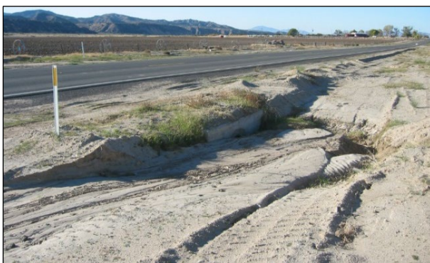
Figure 2.8: Example of blocked side drains and culvert.
