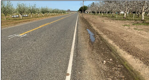
Figure 3.26: Poor drainage associated with absence of paved shoulders and side drains.
