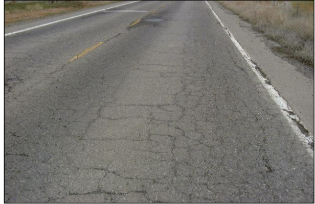
Figure 3.2: Severe fatigue cracking.
