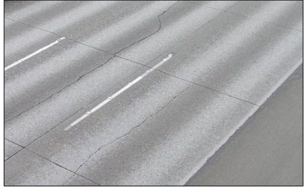
Figure 3.17: Longitudinal cracks on jointed plain concrete slabs.
