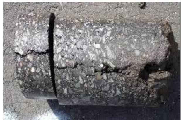
Figure 3.45: Debonded asphalt concrete with full-depth reflective crack.
