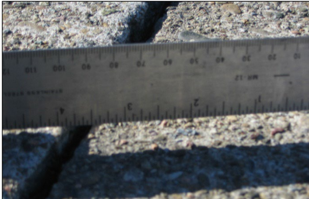
Figure 3.18: Faulting on jointed plain concrete slabs.
