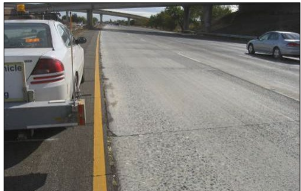
Figure 3.21: Polished surface and loss of texture on jointed plain concrete pavement.
