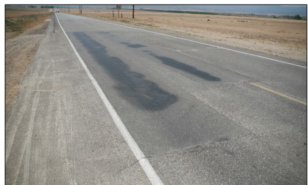
Figure 3.35: Bleeding in digout repairs.
