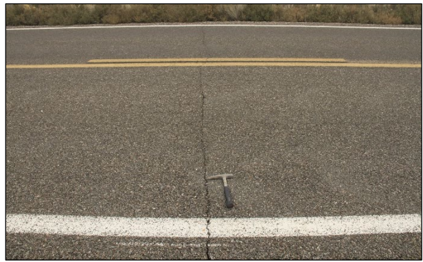
Figure 3.4: Low- temperature cracking.
