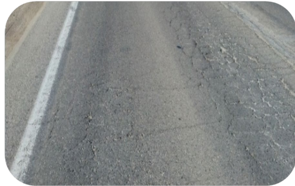
Alligator B Cracking
