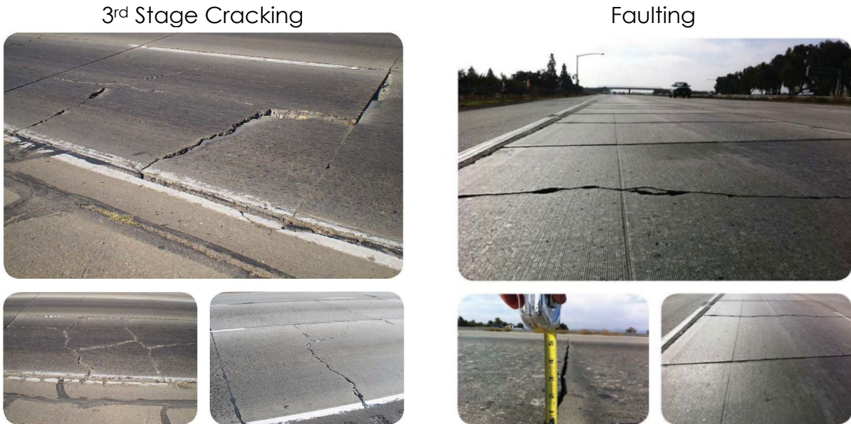
FIGURE 4. EXAMPLES OF DISTRESS FOR CONCRETE PAVEMENT
