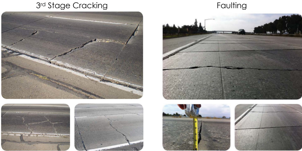
FIGURE 4. EXAMPLES OF DISTRESS FOR CONCRETE PAVEMENT
