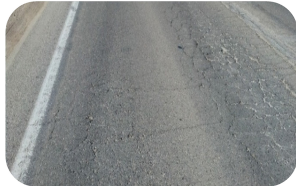
Alligator B Cracking
