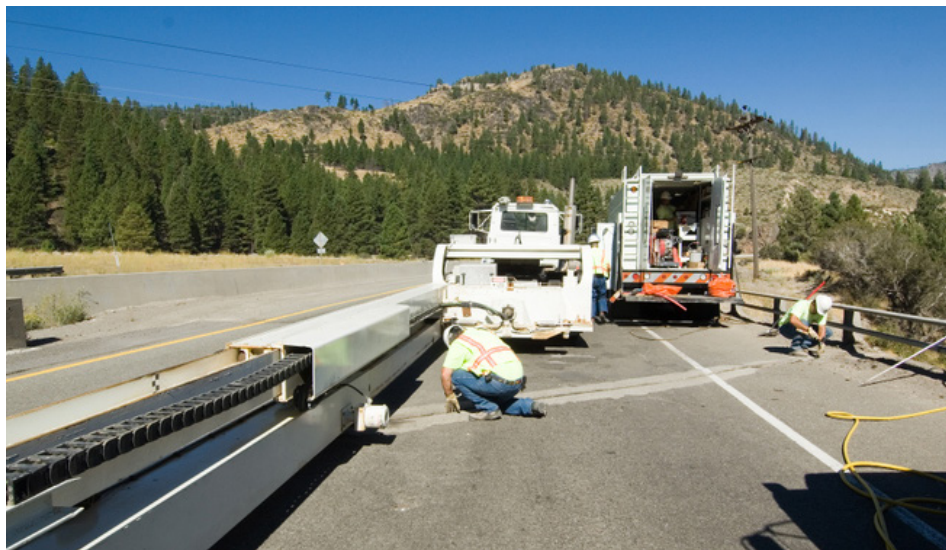
Maintenance workers using the Balsi Beam protection system on a bridge repair.
