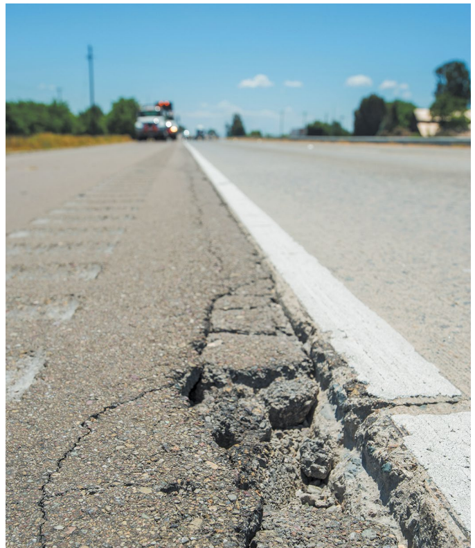
This pothole developed between the asphalt concrete shoulder and Portland cement concrete pavement. Repairs were made.
