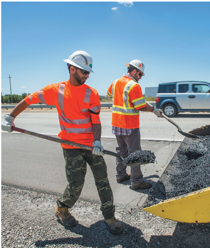
Maintenance Division crews in Stockton-based District 10 repair a pothole with patching material on Interstate 5 outside Lodi.
