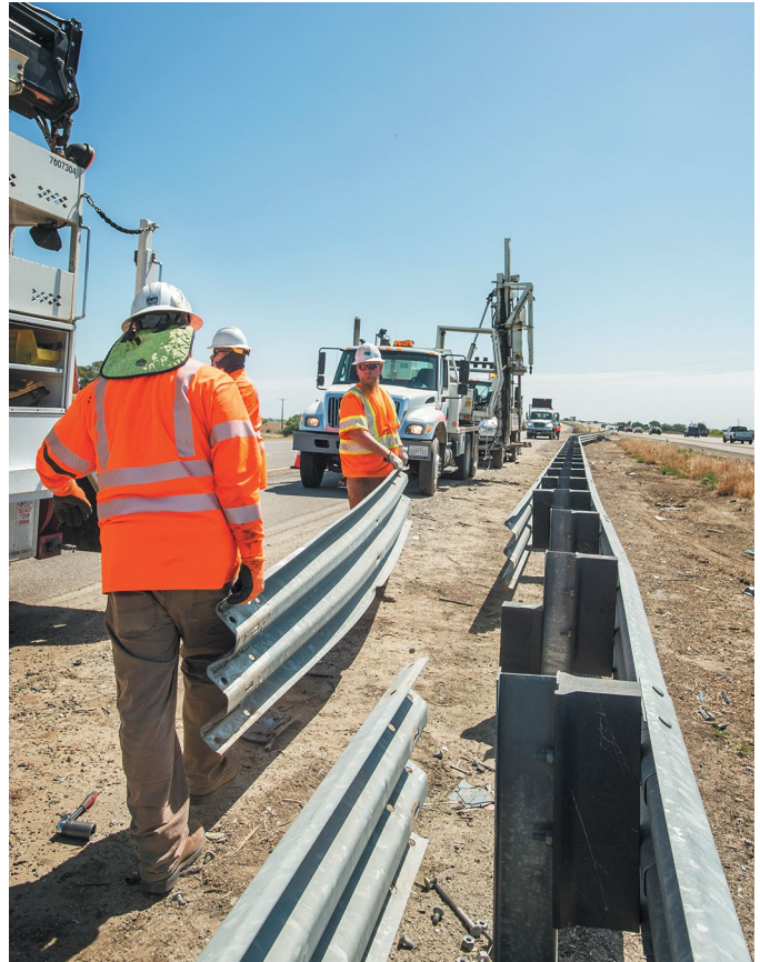
Maintenance crews replace tri-beam guard rails in the median of Interstate 205 near Tracy. There will be $50 million spent on guard rail repairs throughout the state starting in late fall.
