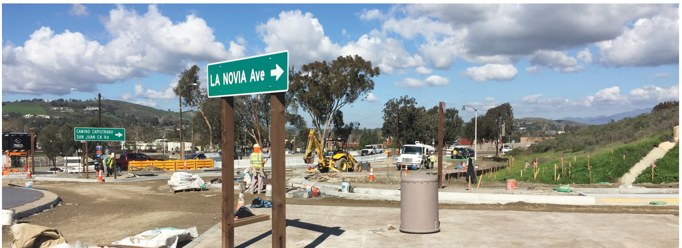
The roundabout project in San Juan Capistrano had to be completed in eight stages, with ramp closures, street closures, and detour maps prepared to alleviate traffic impacts on drivers. The work took 10 months, and the $1.6 million roundabout opened to traffic in April 2017.
