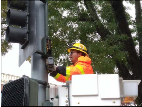
(c) Drilling hole in the small wire box on the signal pole
