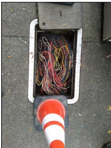
(a) Wire Cabinet beside the Signal Pole
