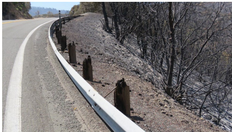
FIRE AFTERMATH ON CULVERTS AND GUARDRAIL, DISTRICT 1
