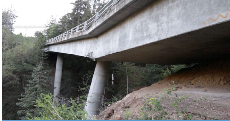
US 1 PFEIFFER CANYON DAMAGED BRIDGE, DISTRICT 5
