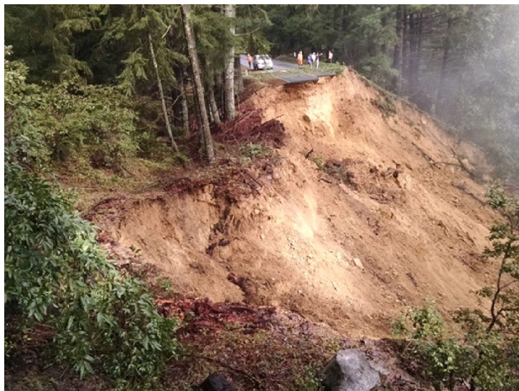
SR 35 WASHOUT, DISTRICT 5
