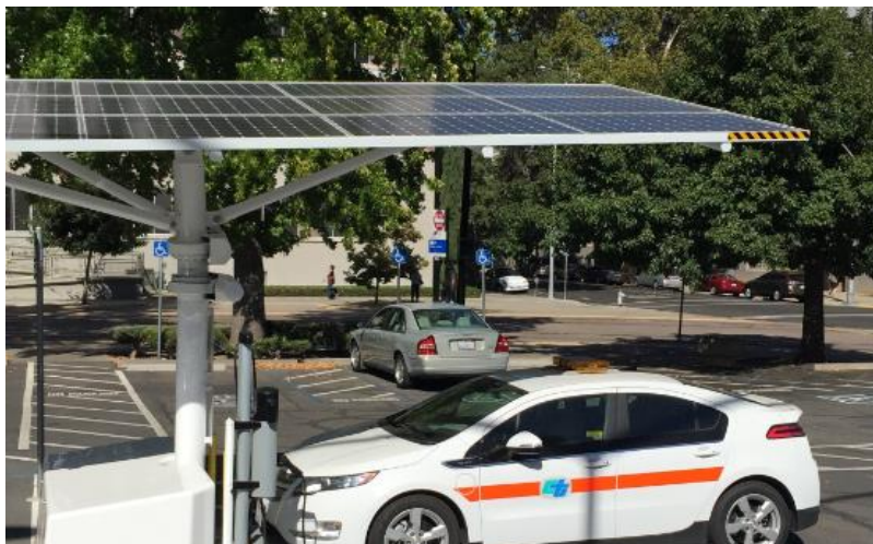
Solar powered EV charging station at Caltrans Headquarters
